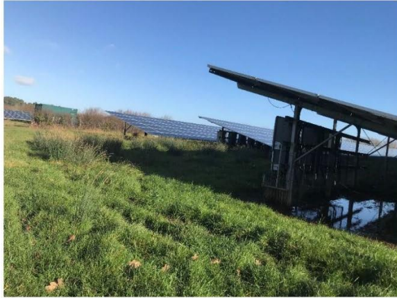
Examples of Localised Drainage Issues/ No Grass Under Panels
